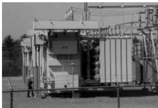
Figure 2: 115kV to 13.8kV AC Transformer
