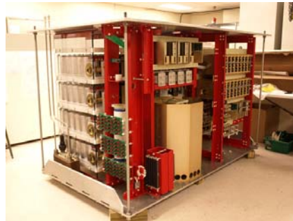
Fig. 6. Long pulse ILC Marx modulator in final stages of completion at DTI.
